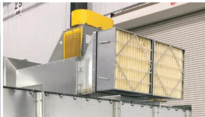
REDUNDANT FILTERS MERV 14 rated
